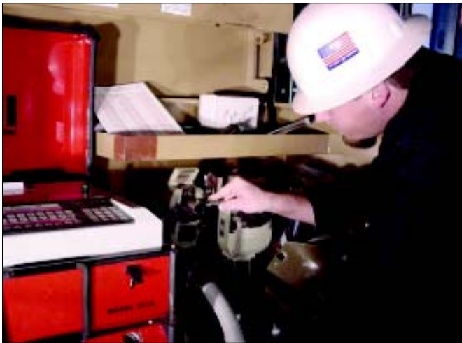
Figure 2. Welding operator installs an electrode in the orbital weld head which is connected to an orbital welding power supply. A water cooling unit is situated beneath the power supply. Photo courtesy of Pro-Tech Process, Inc.
